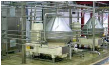
Cold Pressed Peel Oil Recovery
